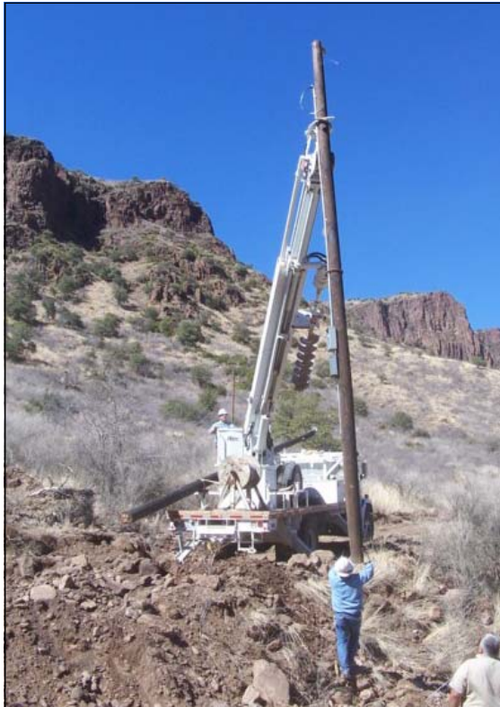
Power Line at Circle H
